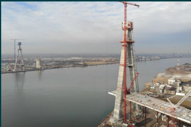
Gordie Howe International Bridge , Windsor, Ontario, Canada to Detroit, Michigan, U.S. PPP Lead Designer for Bridging North America on behalf of Windsor-Detroit Bridge Authority
