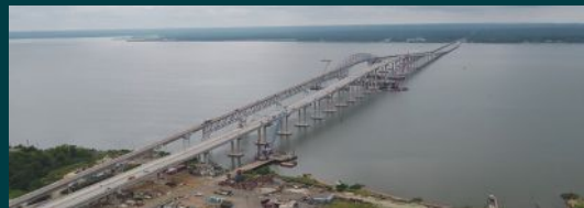
New Nice/Middleton Bridge , Newburg, Maryland to Dahlgren, Virginia, U.S. Design Build EOR for Skanska-Corman-McLean
